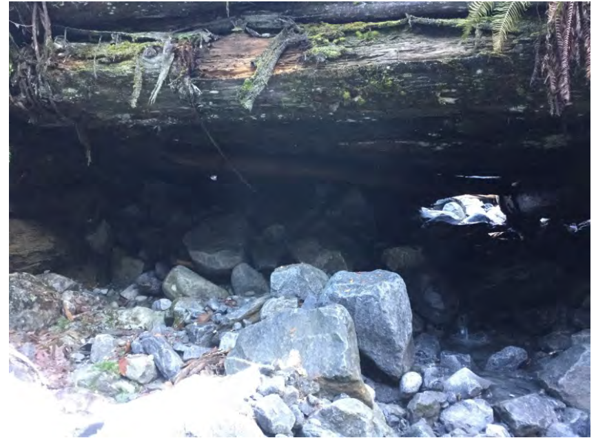
Debris aggrading under bridge
